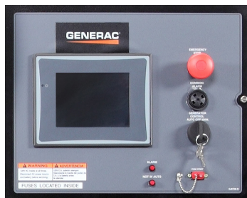
G-Panel (PM-DCP) Control Panel
